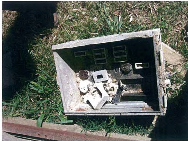
Photograph 12: Switchboard constructed from suspected ACM.
