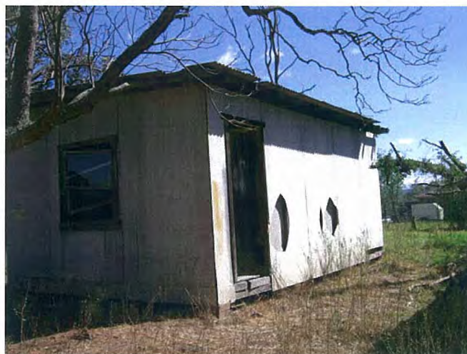
Photograph 15: Shack constructed of suspected ACM.
